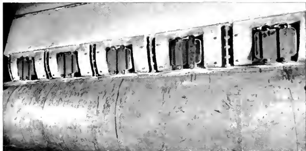
At left, hand holes for cleaning fitted into the shell casing of the watertube boilers on the President Pierce . Below, general view of the after fire room on the President Pierce , showing four furnace fronts and twenty T-4 burners.
